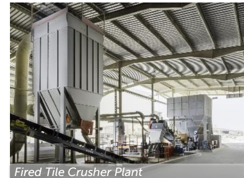
Fired Tile Crusher Plant
